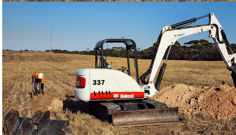
Images: Geotech sample pit investigation works at Riverbend Energy Hub site near Taillem Bend
